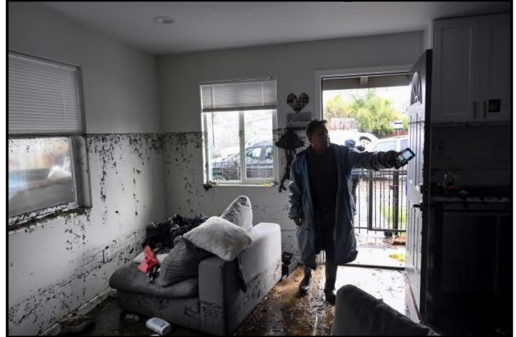
Tony Blas points to the water line inside his home that flooded during a rainstorm Monday, Jan. 22, 2024, in San Diego. (AP Photo/Denis Poroy)
