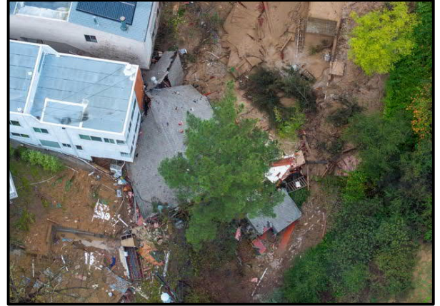
An aerial image of a home destroyed by a landslide in Los Angeles, California on Monday. AFP via Getty
